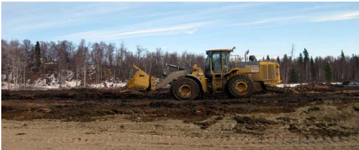
Ground preparation is underway for construction of the Goose Creek Correctional Center at Point Mackenzie. The department's newest facility is scheduled to open in 2012. (photo courtesy RISE Alaska)
