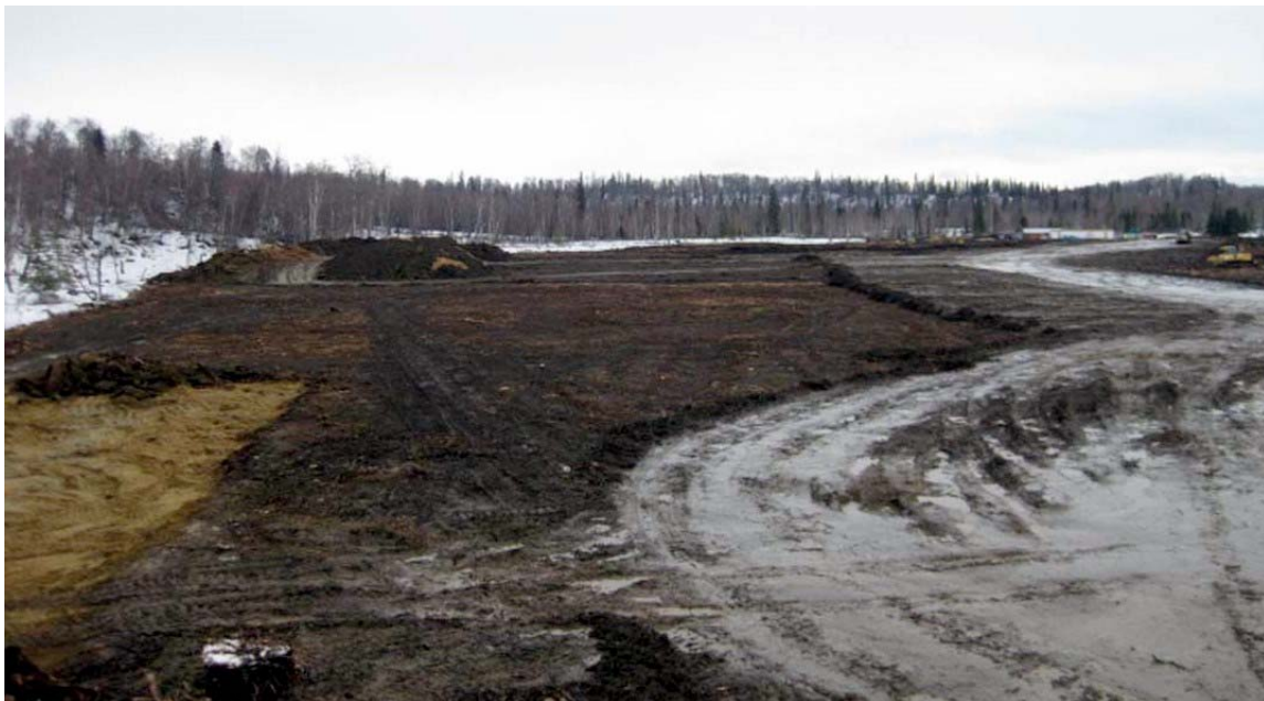
Ground preparation has begun on the $240 million Goose Creek Correctional Center at Point Mackenzie. The official groundbreaking will be in June. (photo courtesy RISE Alaska)
